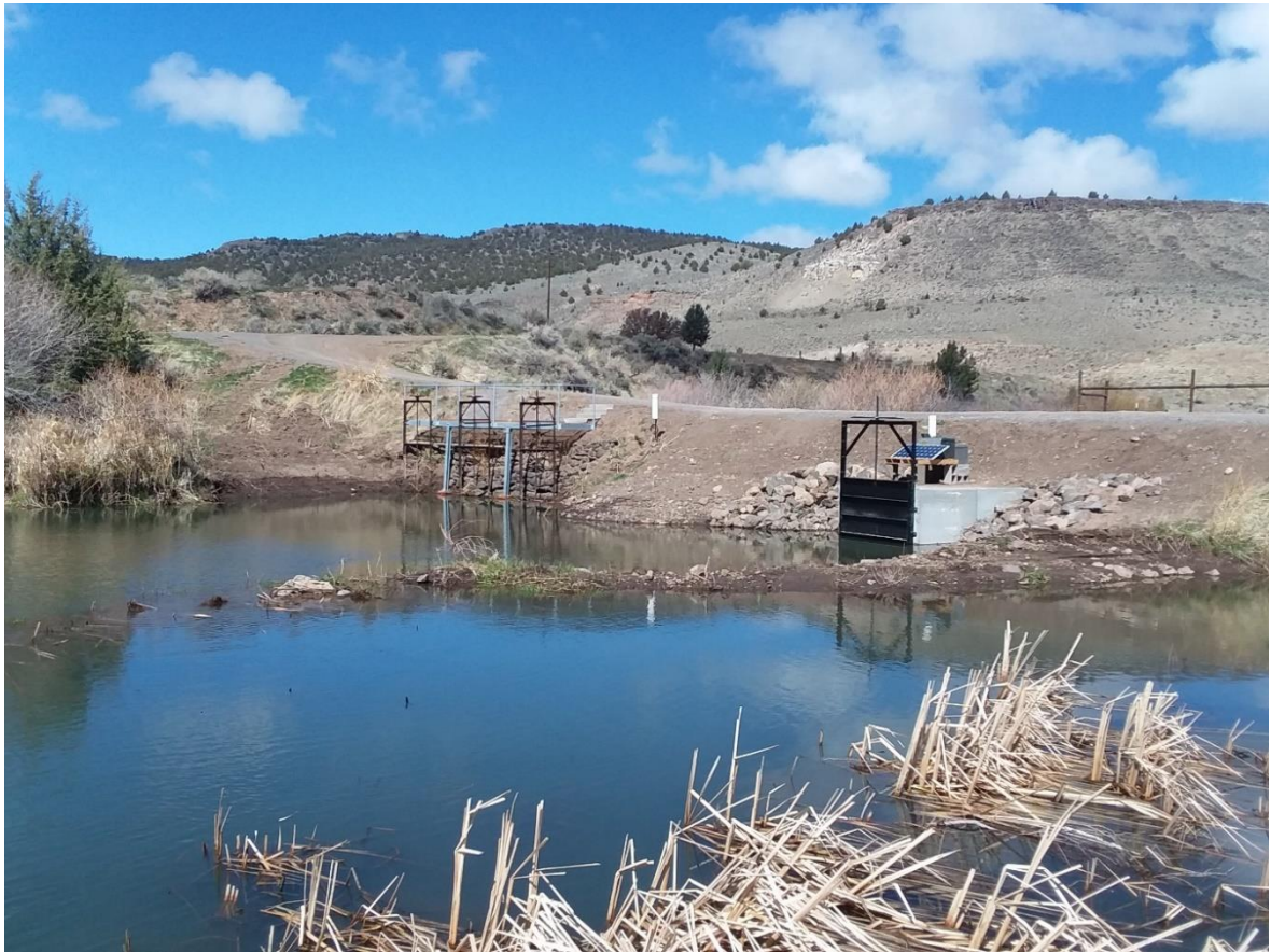
Photograph of the MC Diversion showing old culverts and new box culvert.
