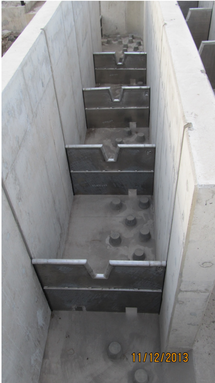
Figure 5. Photograph of the weir panels and artificial boulders in the Rookery Diversion passage structure on lower Honey Creek.
