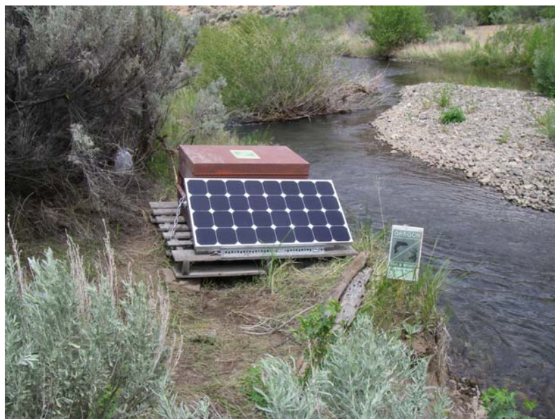
Figure 6. PIT tag antenna installed in Twentymile Creek. Photo shows the box containing the multiplexer and batteries and the solar panel. The flat plate antenna wires are in the stream channel.
