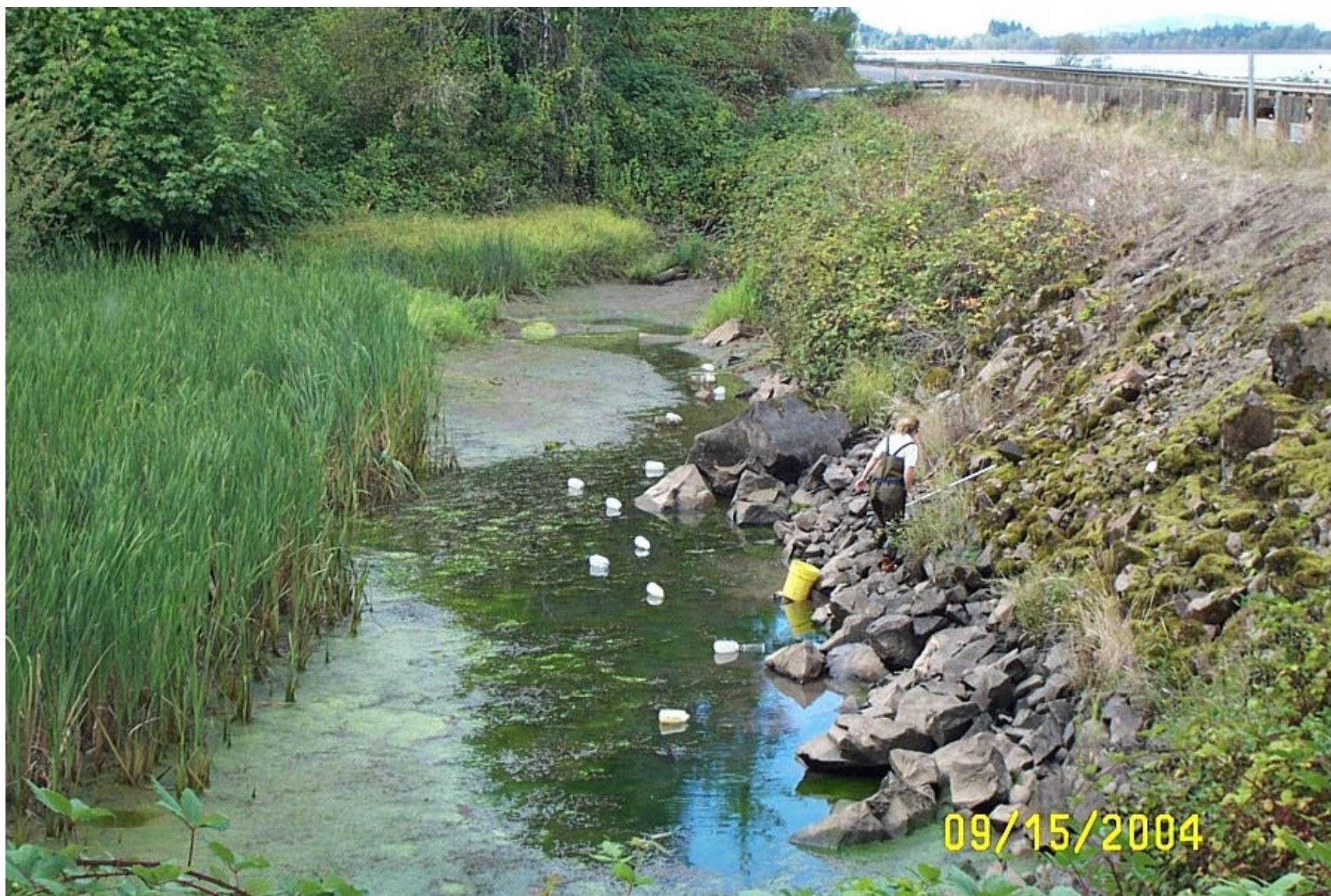
Figure 8. Low water levels observed in the Dexter alcove “The Pit” on September 15, 2004. Note the limited wetted areas between the mud flats and the rip rap. The culvert is in the background. Dexter Reservoir elevation was 690.2 feet on this date.
